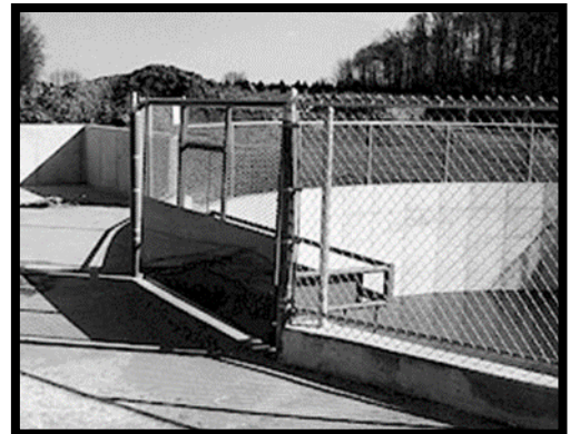
Manure pit push-off fence and bump rail example.
